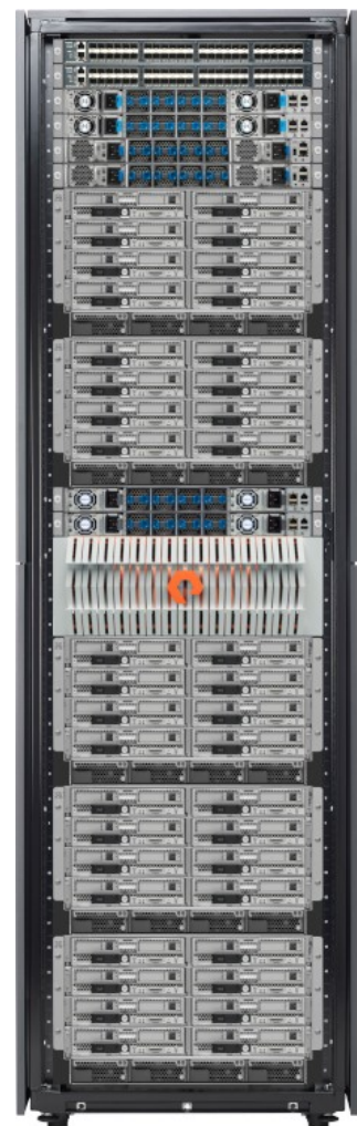
FIGURE 1. FlashStack with FlashBlade
