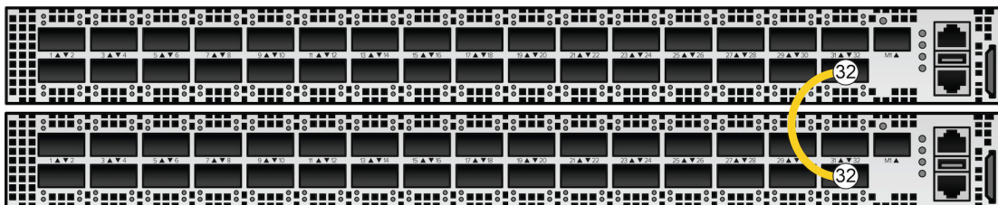
Figure 4.5 Connect EV Cable to Port 32 on XFM-8400 Modules
